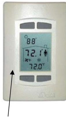
Room Temperature Control and display
